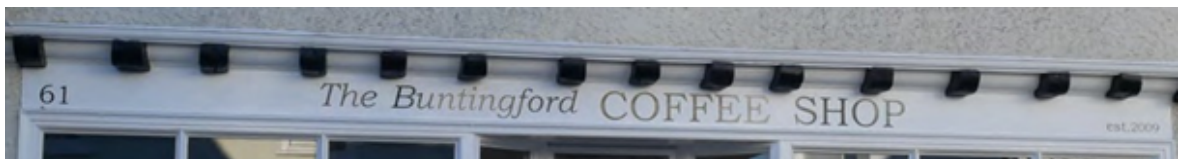
Figure 24 - Various sign and fascia issues
